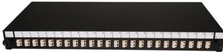
Sliding patch panel equipped with 24 LC duplex multimode connectors.
